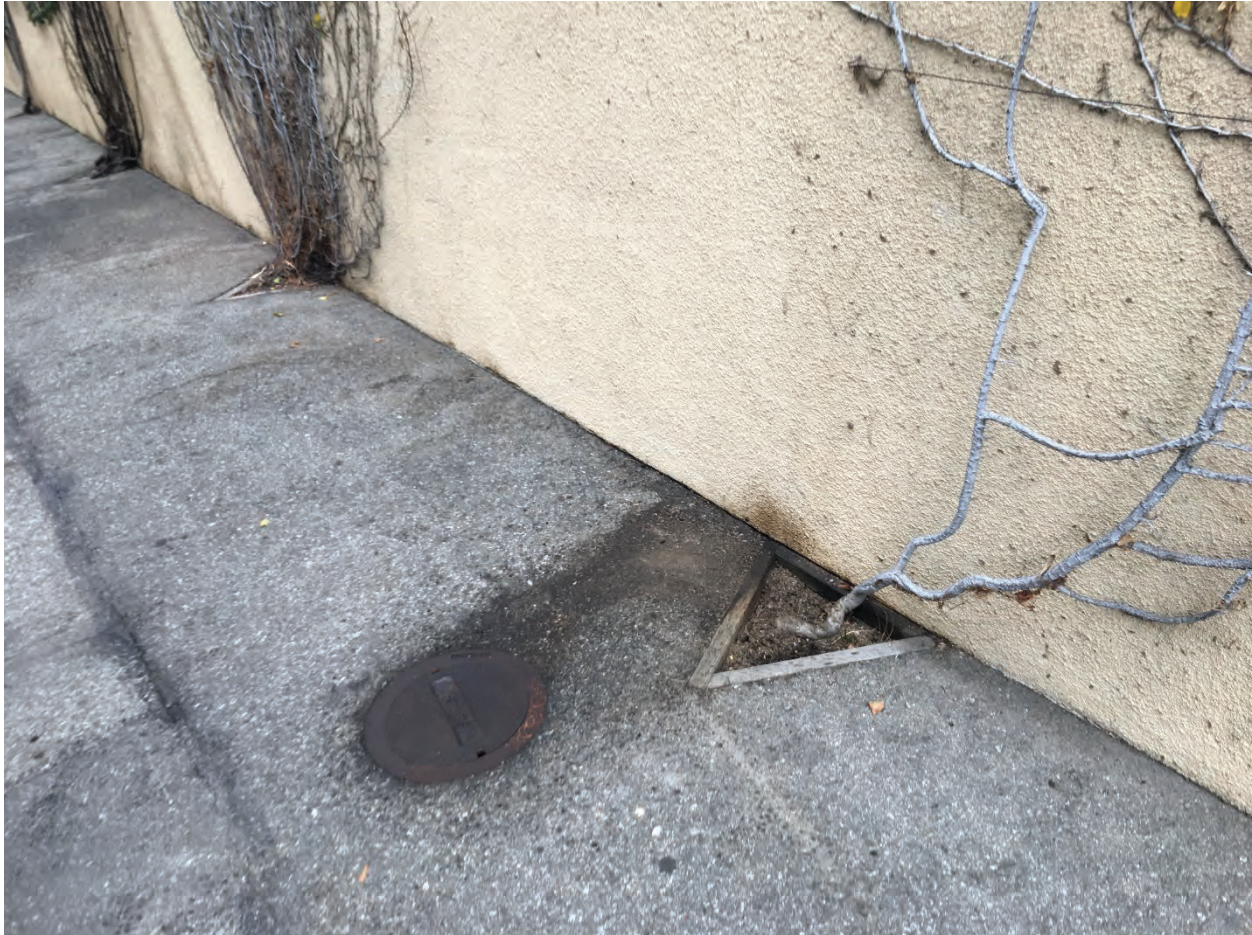
Figure 7. The leaks were in between these four vines pictured.
