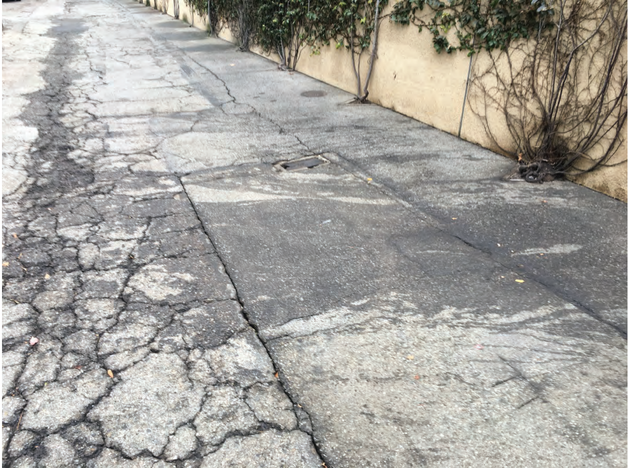
Figure 3. Staining shows point source with most discharge as well as lateral extent into the alley
