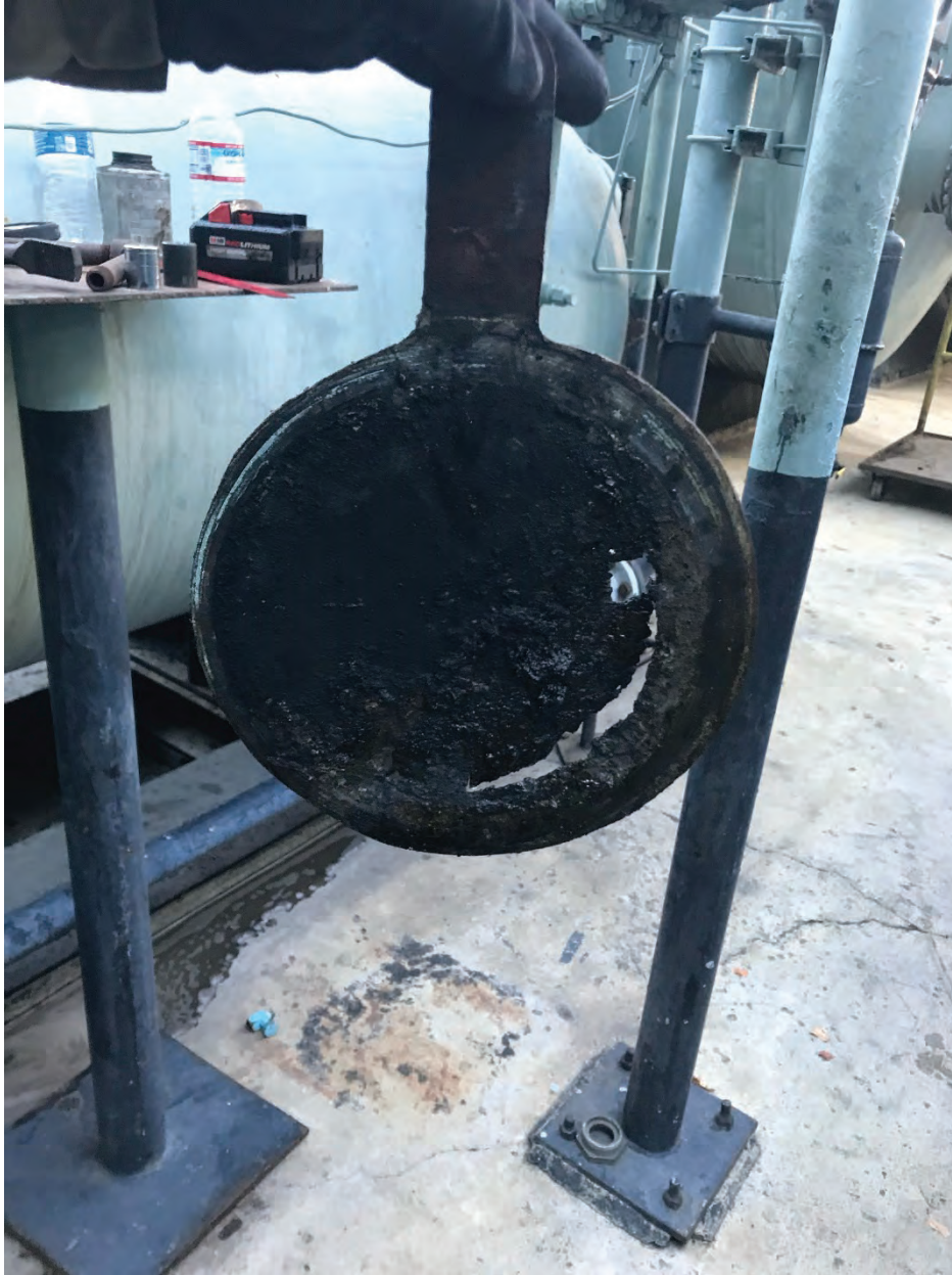
Figure 12. This picture shows the corroded blind slip that was the root cause of fluid entering the out of service pipeline that is buried near surface expression of the leak in the alley.
