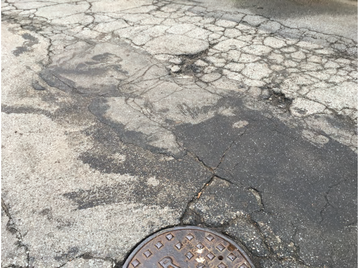
Figure 5. shows leaked fluid migration extent
