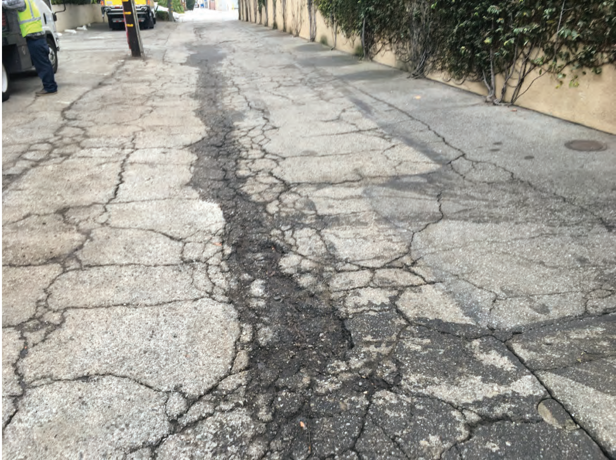
Figure 2. This photo shows the area affected by the leaked fluid. The fluid pooled in the center of the alley and travelled west down the alley. It was reported that the fluid was removed with absorbent material and the ground was steam cleaned. At the time of the photo, there was no oil present. What is seen here is staining. There are no sewer or drainage systems affected. Visual staining was present on the alley surface.
