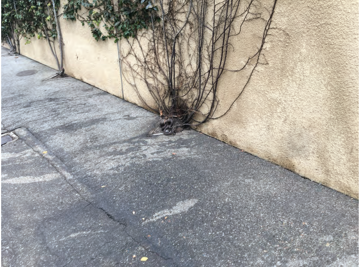
Figure 6. The fluid was extruded through the joint where the building wall met with the asphalt alley. The area shown here was the main location of leaking with minor leaks further east and west in the photo. The area which had leaks was approximately 10 feet in length.
