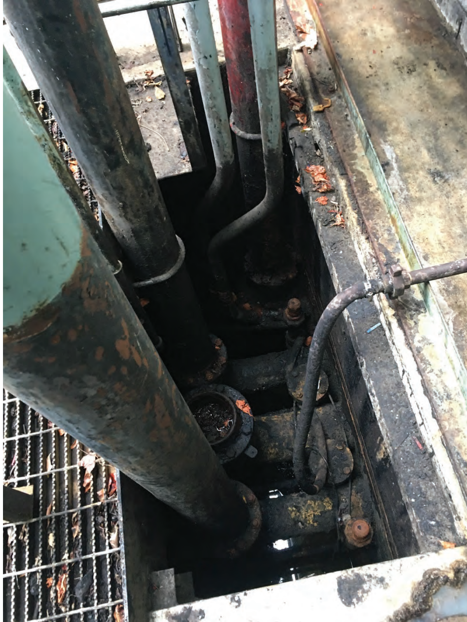
Figure 10. This photo shows the out of service lines entering the cement to run underground to the production facility. The two 6-inch lines were still connected to the pressurized pipeline system but isolated with a "slip blind" that failed.
