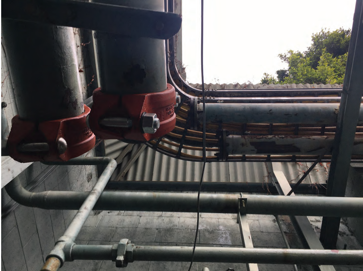
Figure 11. The photo shows the out of service pipelines with red caps having been disconnected from the horizontal pipelines that are still under pressure. At the time of the leak, these two ends were connected and the out of service segment was isolated from pressure with the use of a "blind slip" that was found to be corroded to the point of leaking.
